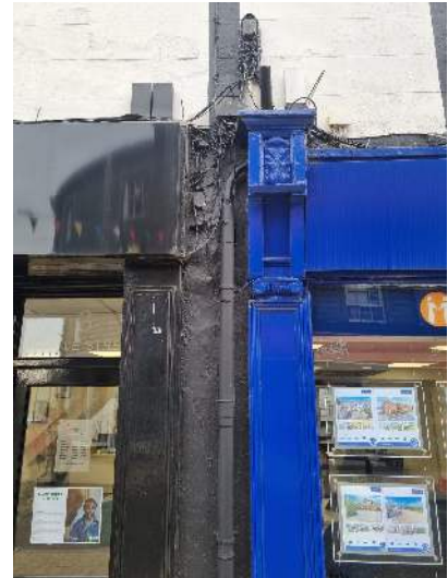
Figure 9 On the left is a fascia of inappropriate material and size, extending over the corbel. On the right is a modest fascia contained by a decorative corbel.
